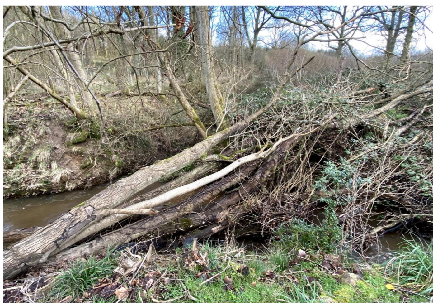
Figure 3: Stroud style leaky barrier, oblique across channel
